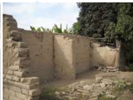
Structural Damage from Earthquakes
